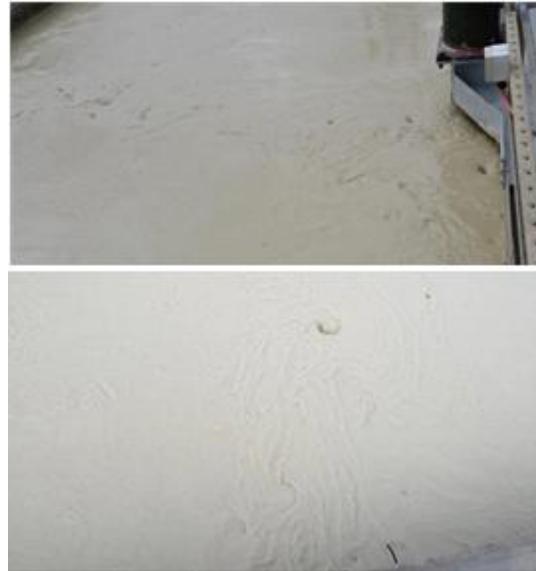
Figure 4: Small Swirls Observed on Site Visit at Central Line
