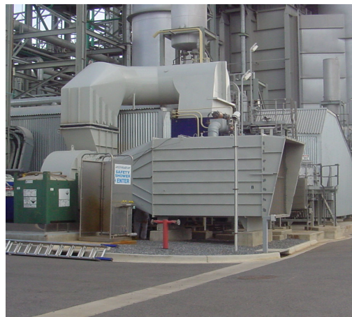
Figure 1: View of the duct system.
