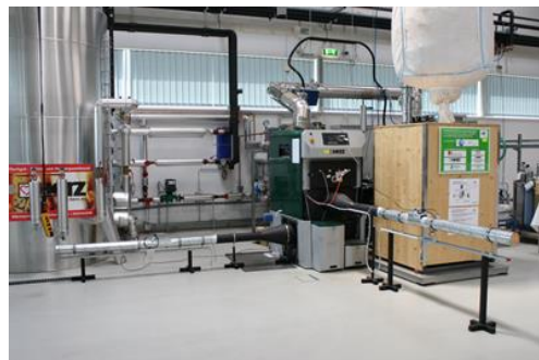
Figure 7: Experimental test rig used for the 100kW wood pellet boiler.
